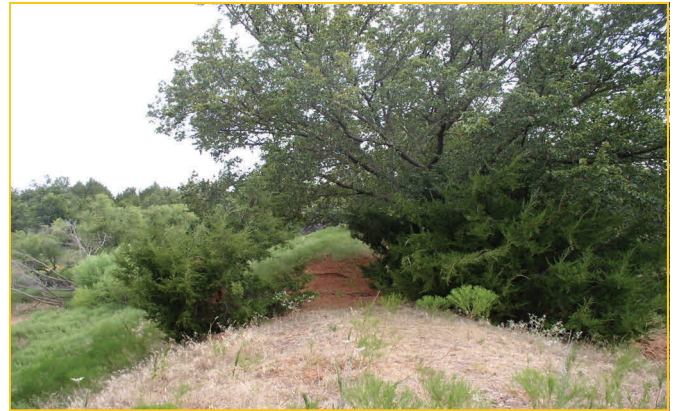
Trees growing on pond dam and in spillway
